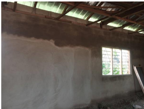
These last four photos show the building plastered and windows installed. I hope you'll notice the electrical wires being connected
